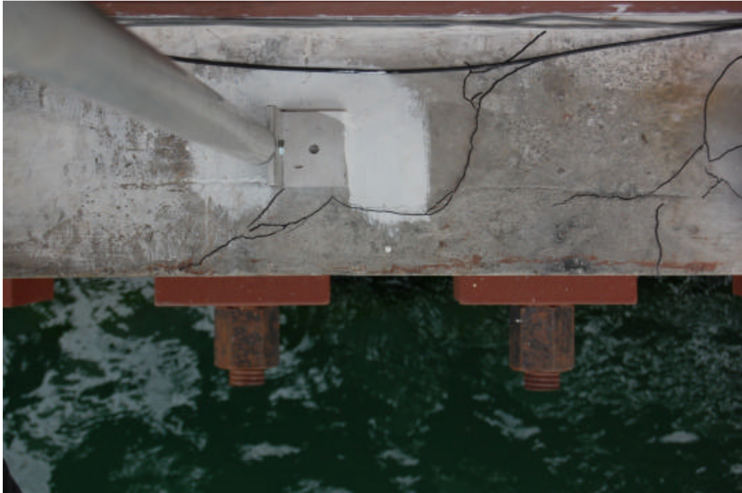
Figure 2.30 - Cracking in Wall below Window Opening Supporting the Reaction Plate
