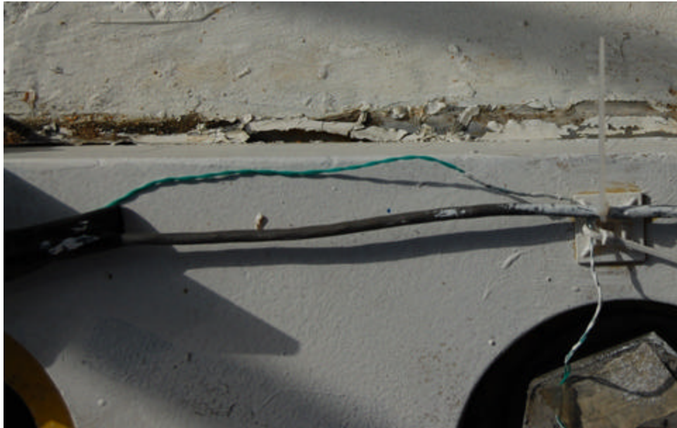
Figure 3.15 - Photograph of Slip Marks of the Bollard
