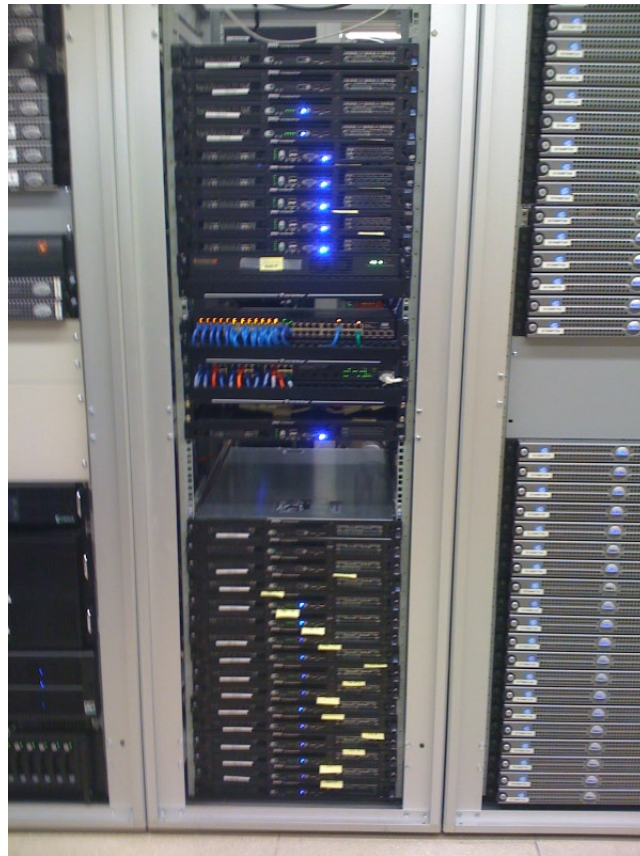
Figure A.1: Our Experimental Data Center
