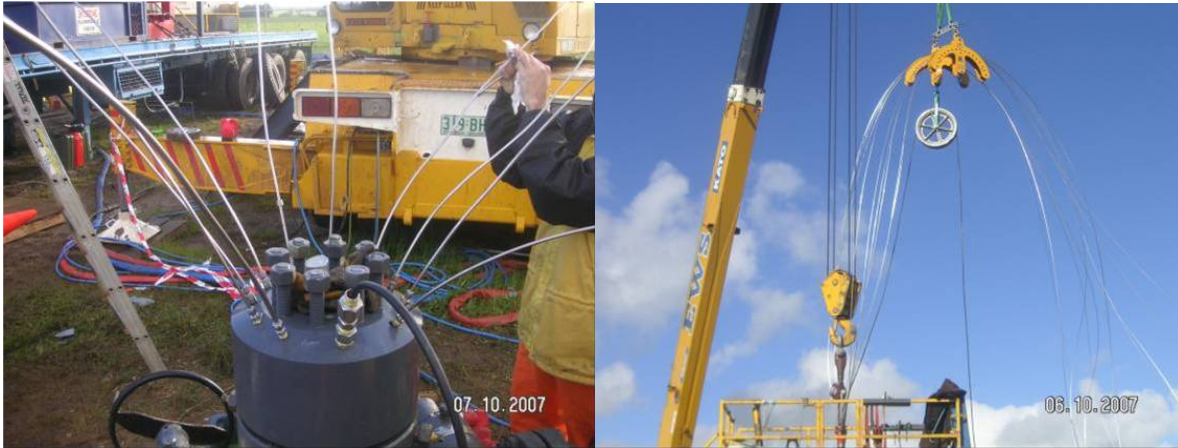
Figure 5. Assembling and deployment of the complete system was a complex and successful operation, these figures show the wellhead with flow tubes and cable connections, while on the right shows control of the u-tubes while inserting the integrated assembly
