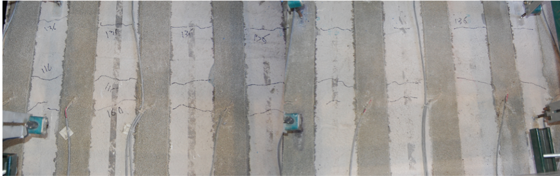
Figure 6.40 Cracking of deck slab at 184 kN (41 kip) per jack- top view of deck
