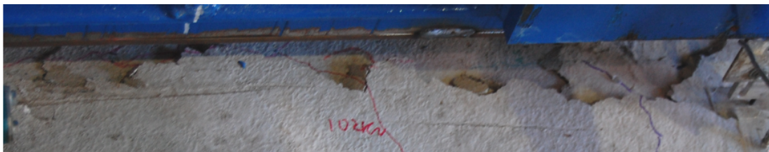
Figure 6.18 Detail of cracking at ultimate capacity in central section of deck near loading beam
