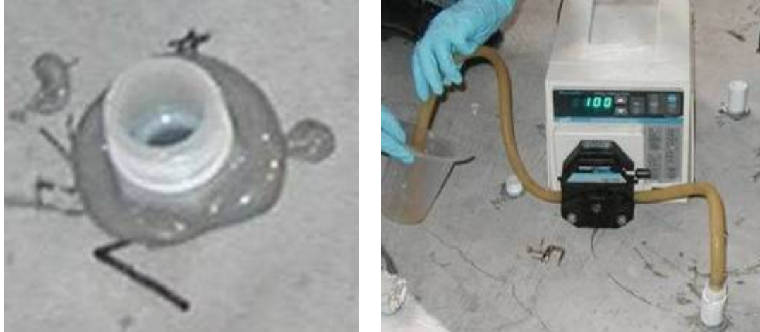
Figure 4.3 Injection port in top of deck and setup used to inject resin into deck
