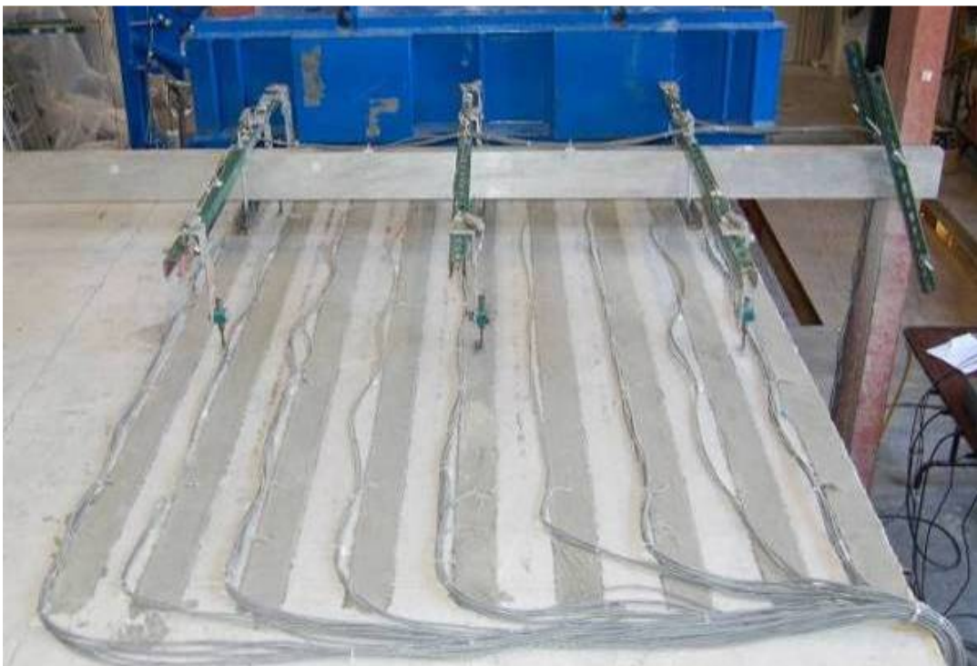
Figure 6.39 Side view of completed installation of CFRP strips with full instrumentation setup
