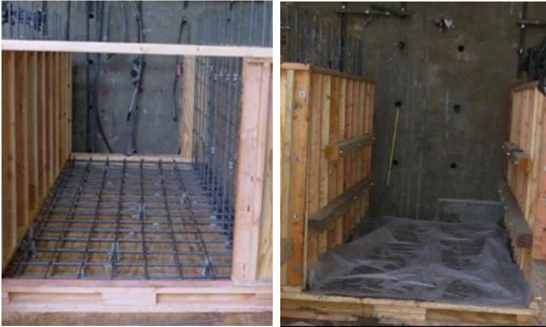
Figure 3.6 Lower portion of the box girder bridge before and after casting of concrete
