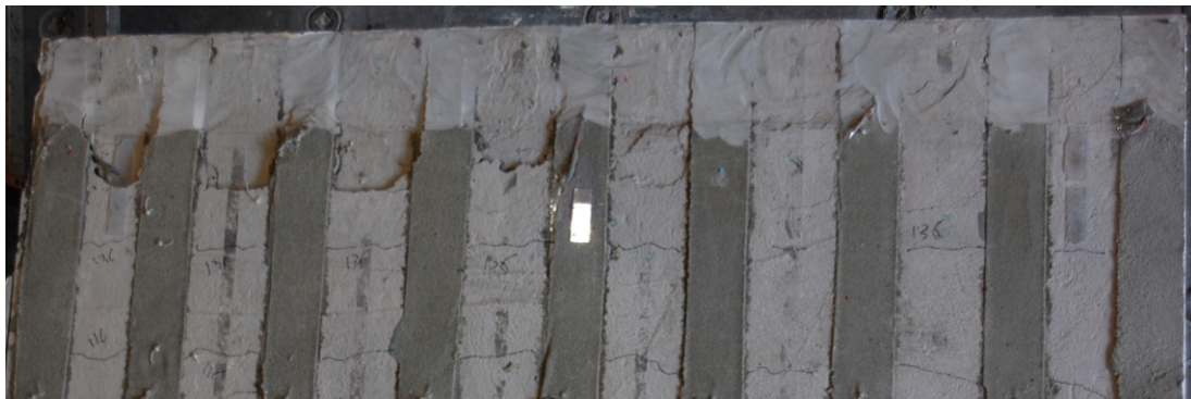
Figure 6.66 Detail of cracking observed at ultimate capacity- top view of FRP rehabilitated deck
