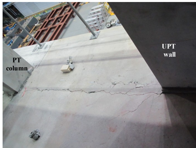
Figure 5-17 Damage in slab at location of UPT beams at end of tests; picture courtesy of T. Nagae
