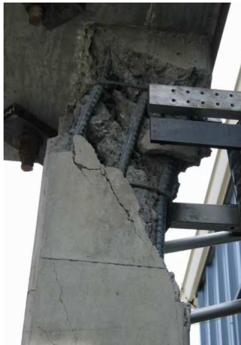
Figure 3.53: Top Damage Detail (Test 7)
