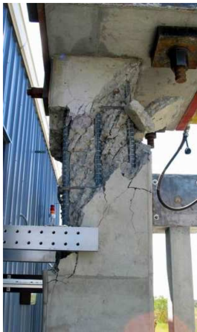
Figure 3.23: Damage Pattern Top Right (Test 3)
