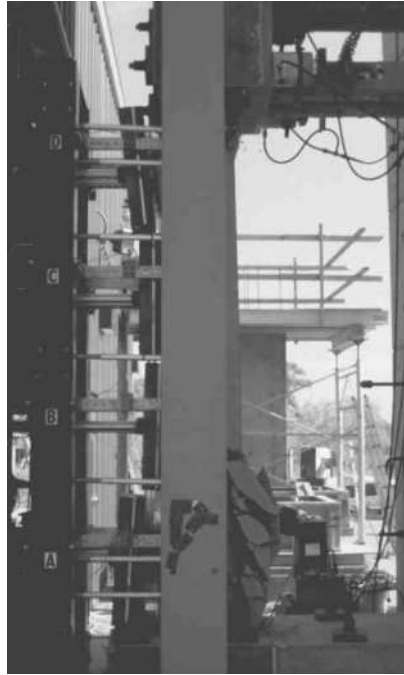
Figure 3.62: Advanced Damage (Test 8, 53.0 ms)
