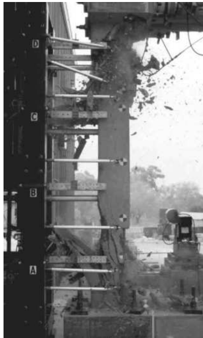
Figure 3.50: Advanced Damage (Test 7, 350 ms)
