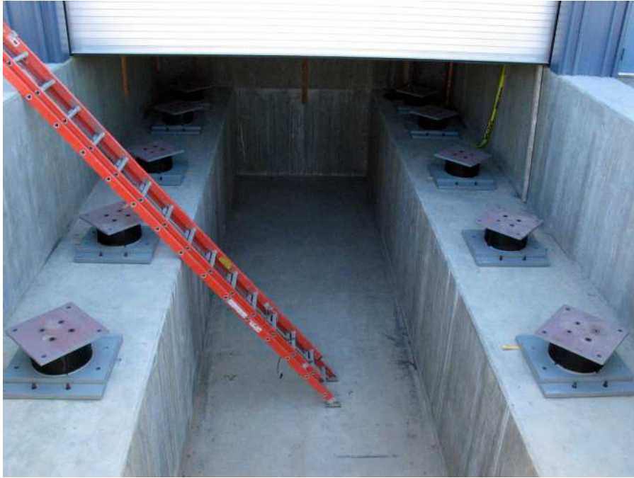
Figure 2.19: Isolators in Position (10 Aug, 2003)
