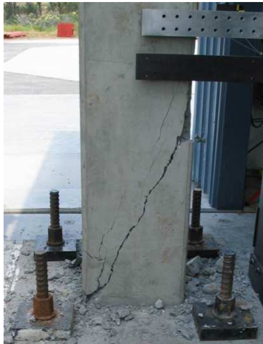
Figure 3.25: Damage Pattern Bottom Left (Test 3)
