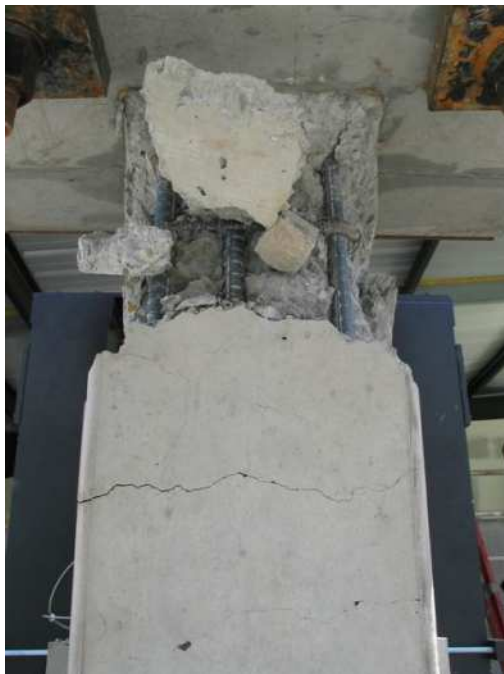
Figure 3.22: Damage Pattern Top Rear (Test 3)
