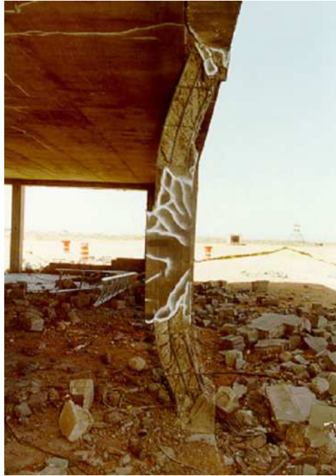
Figure 1.13: As-Built Specimen Post-Test (DB 6) [43]
